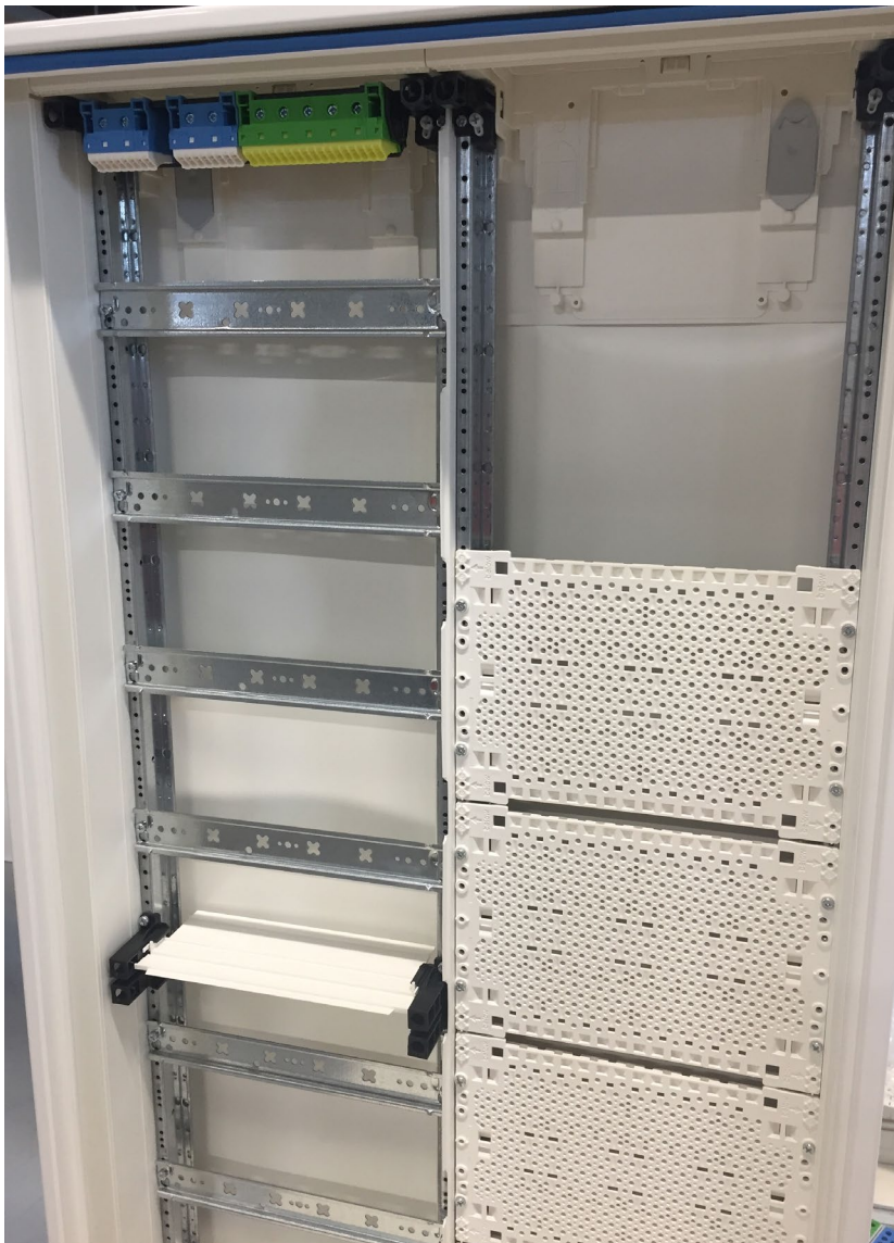
Cabinet with installed partitions
